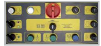
• Quadro comando • Control panel
